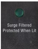
Surge Protection module
