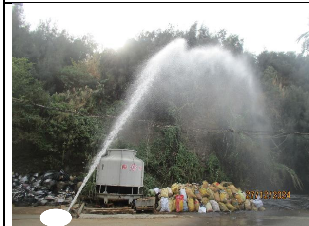
Fire hydrant testing
