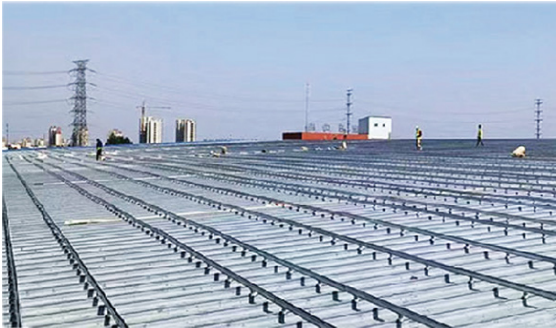
Fudao Logistics JD.com Warehouse Photovoltaic Power Station in Shijiazhuang, Hebei Province 2MW Project
