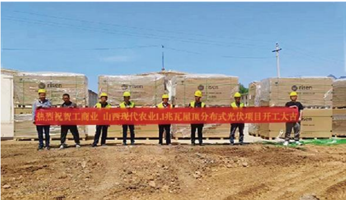
Wutaishan Modern Agricultural Park Photovoltaic Power Station in Shanxi Province 1.1MW Project
