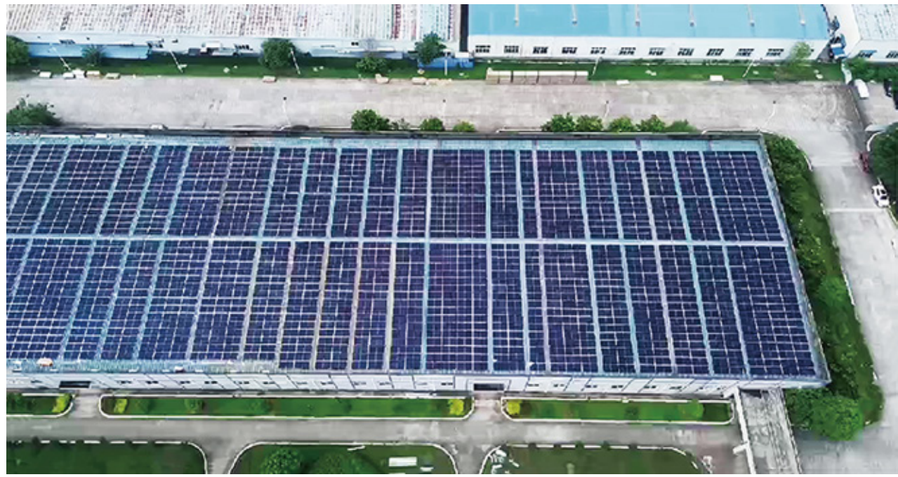
Chengdu Zhongda Soft Plastic New Materials Co., Ltd. Distributed Photovoltaic Power Station 3.23MW Project
