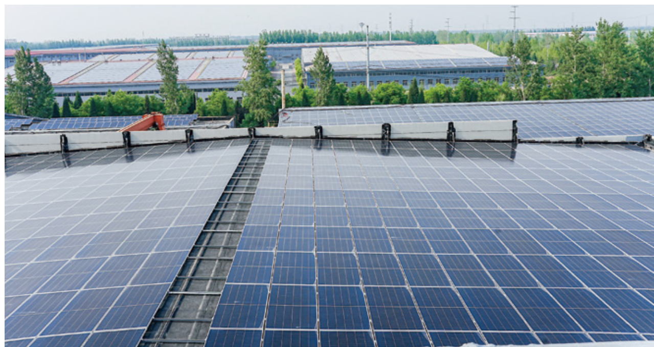
Hebei Taineng Hongsen Medical ABC Distributed Photovoltaic Power Station 12MW project
