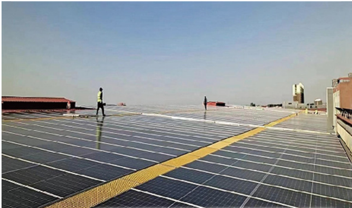
Poverty Alleviation Photovoltaic Power Station in Zagui Banner, Ulanhot City, Inner Mongolia 300KW Project
