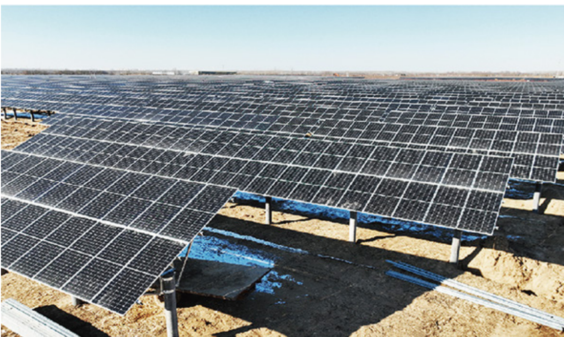
Xingtai Weixian Ground-Mounted Distributed Photovoltaic Power Station 42MW Project
