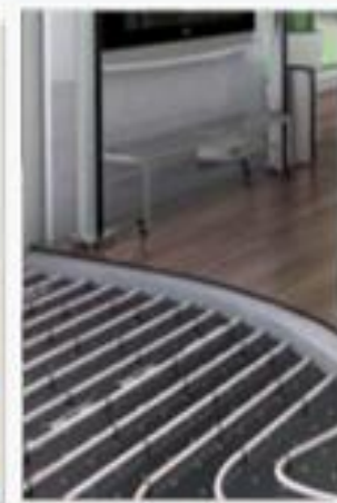
electric heating floor
