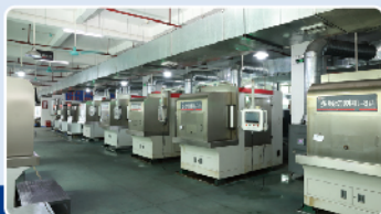
Multi-Wire Cutting Machine 多线切割车间
