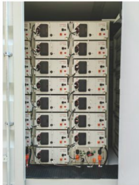
Project Capacity: 3MW/10MWh Project Location: Hebei, China
