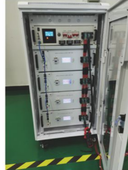
Dusseldorf Germany 5kW+20kWh battery RESS
