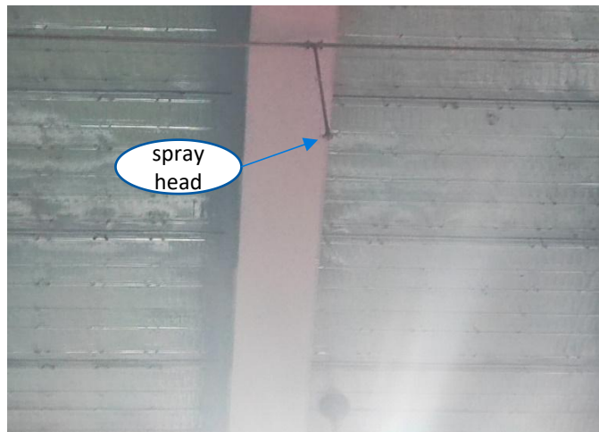
Automatic humidification spray system
