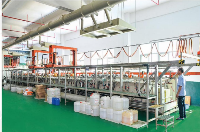
Automatic copper deposition line
