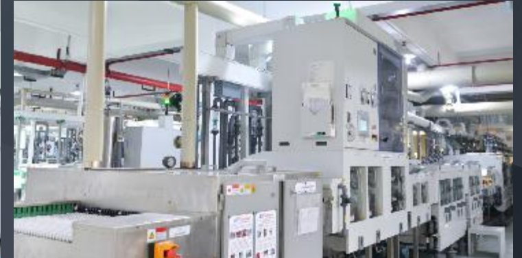
Inner Layer DES (Developing, Etching, Stripping) Line
